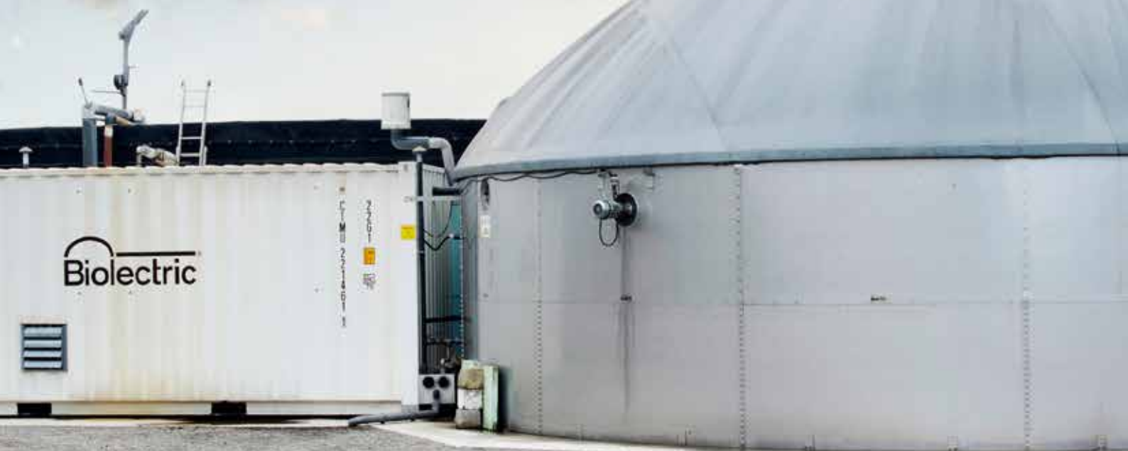
Bioelectric • Combined-heat-and-power biogas installation
