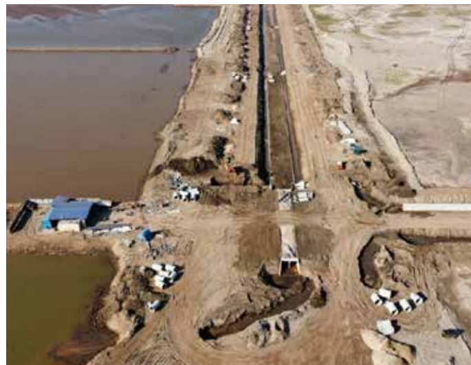
Deep C Holding • Land reclamation and construction of drainage channel at an industrial zone
